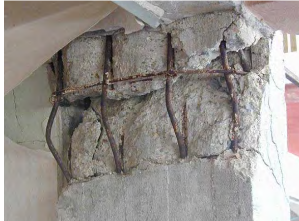
Figure 4.34: Buckling of the steel reinforcement of a reinforced concrete column (Barbat and Cardona, 1999).
